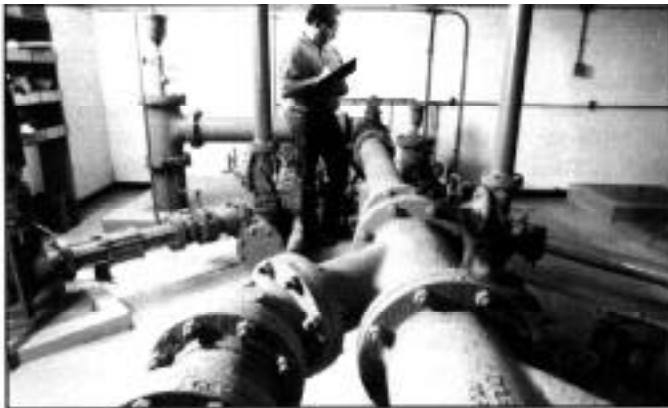
Jim Zeck, chief plant operator at Minnehaha Community Water Corp., takes readings from the system's gauges. Minnehaha, in Dell Rapids, South Dakota, is one of more than 200 rural water systems assisted by CoBank.
